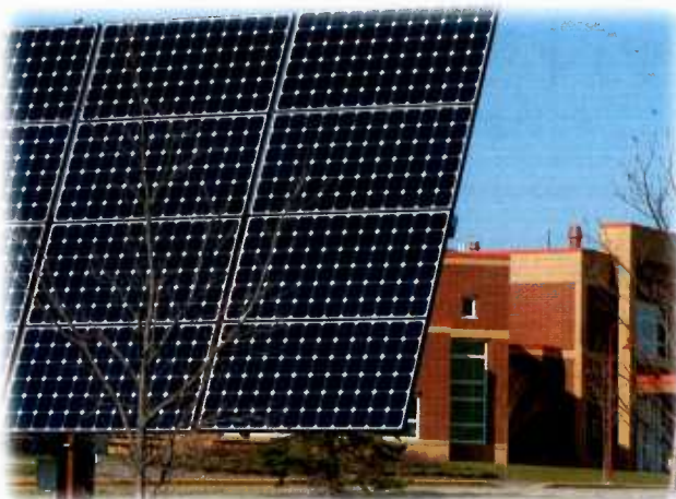
Located at the River Falls High School, this 3.7 kW photovoltaic dual-axis tracker system is estimated to produce 5,236 kWh per year.
